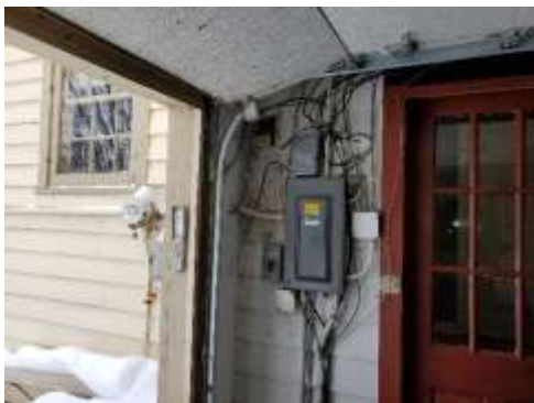
Existing electrical box/wiring
